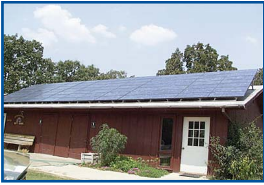
Solar system installed at the Heifer Ranch in Perryville, Arkansas. Photo courtesy of NREL.
